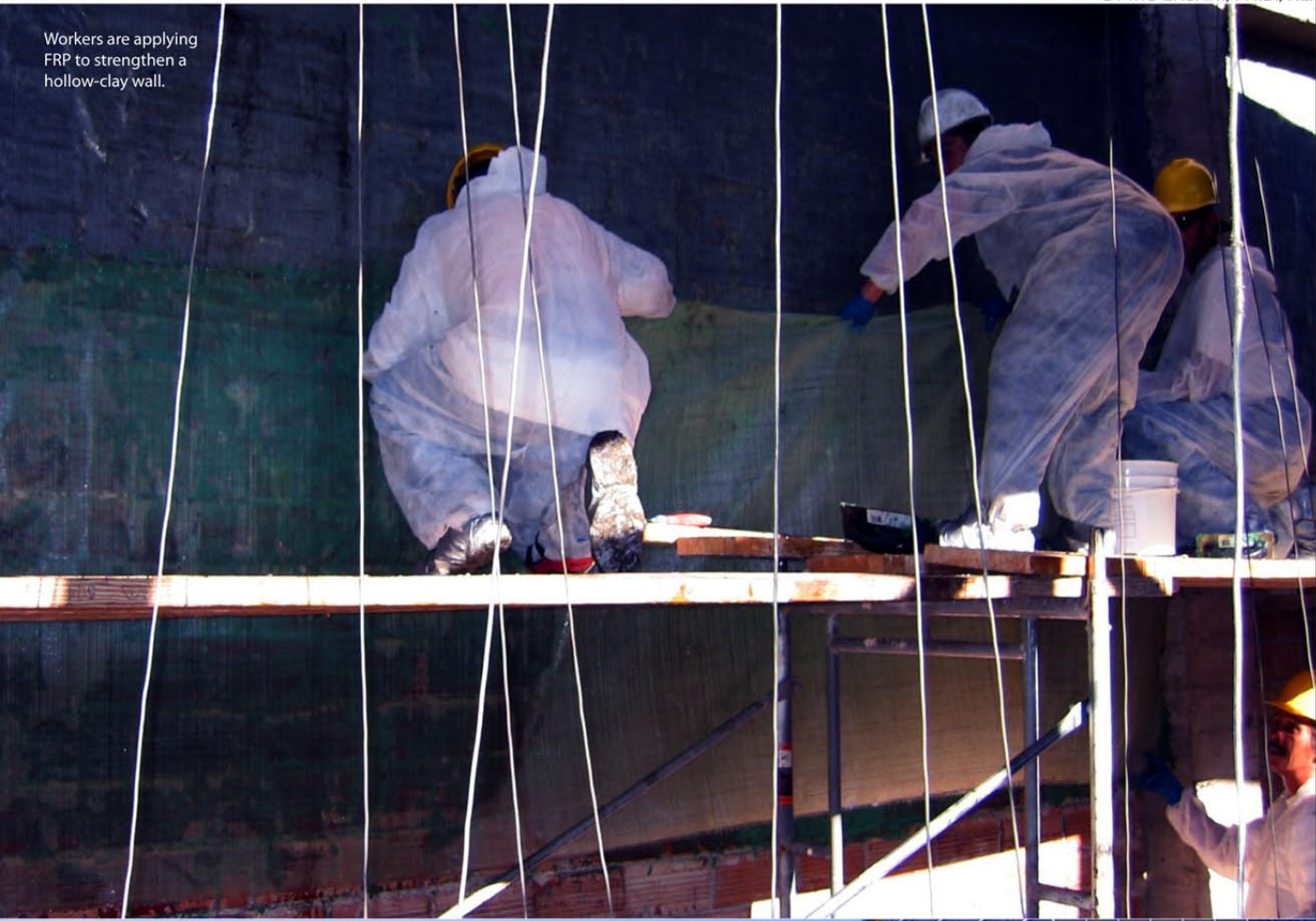
Rolls of fabric constructed with carbon glass fibers are saturated with a special epoxy resin and then bonded to the exterior surface of an unreinforced brick wall and parapet.
